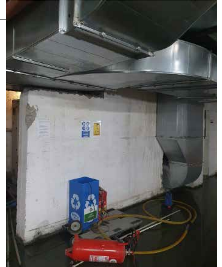
Ventilation system passing through the shear wall!!!
