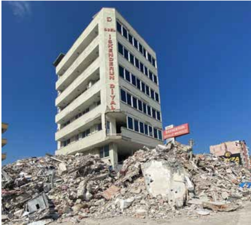
Private Dialysis Center Damaged but standing!
