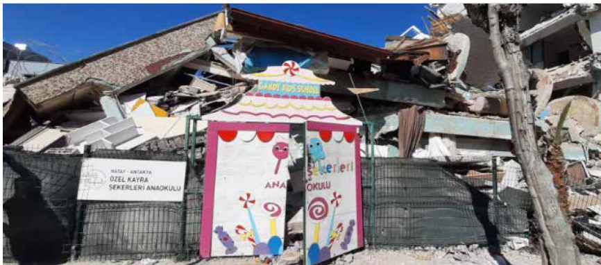
Pancake-style complete collapse
