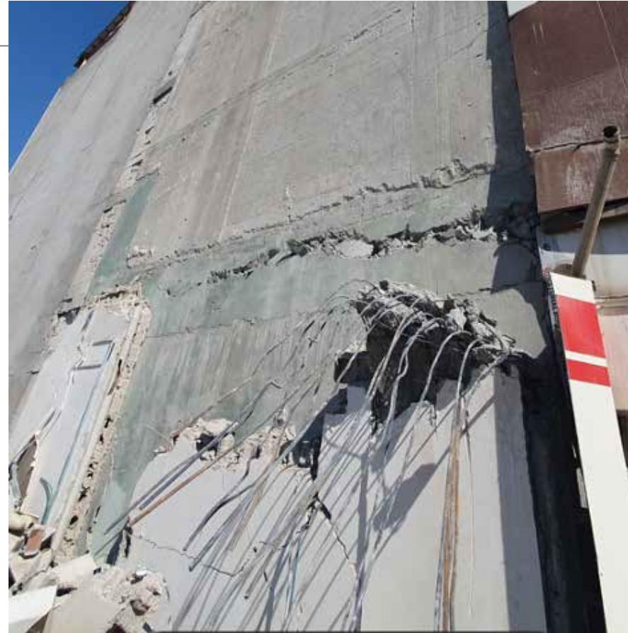
Shear wall damage – exterior view
