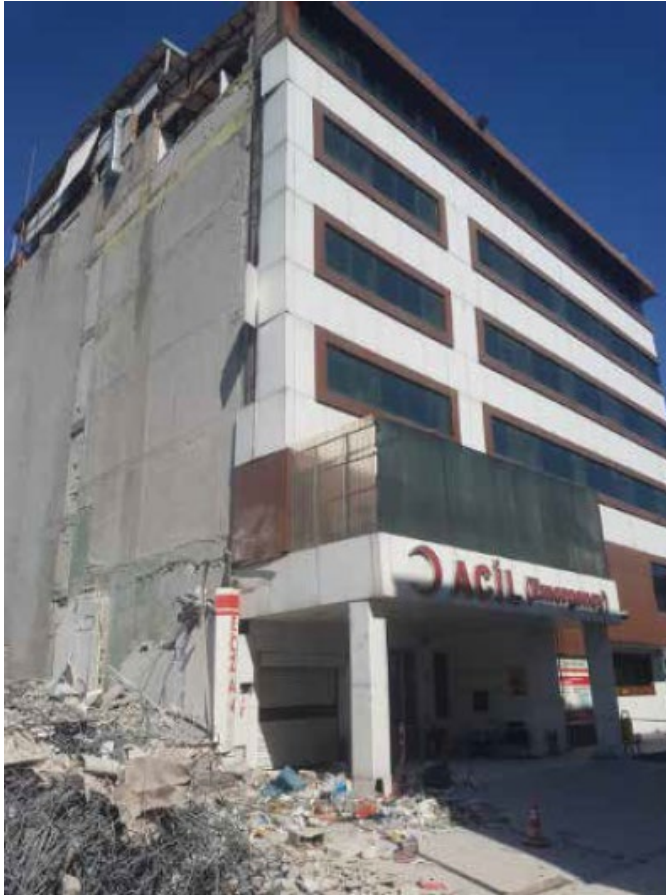
Exterior - next building is collapsed
